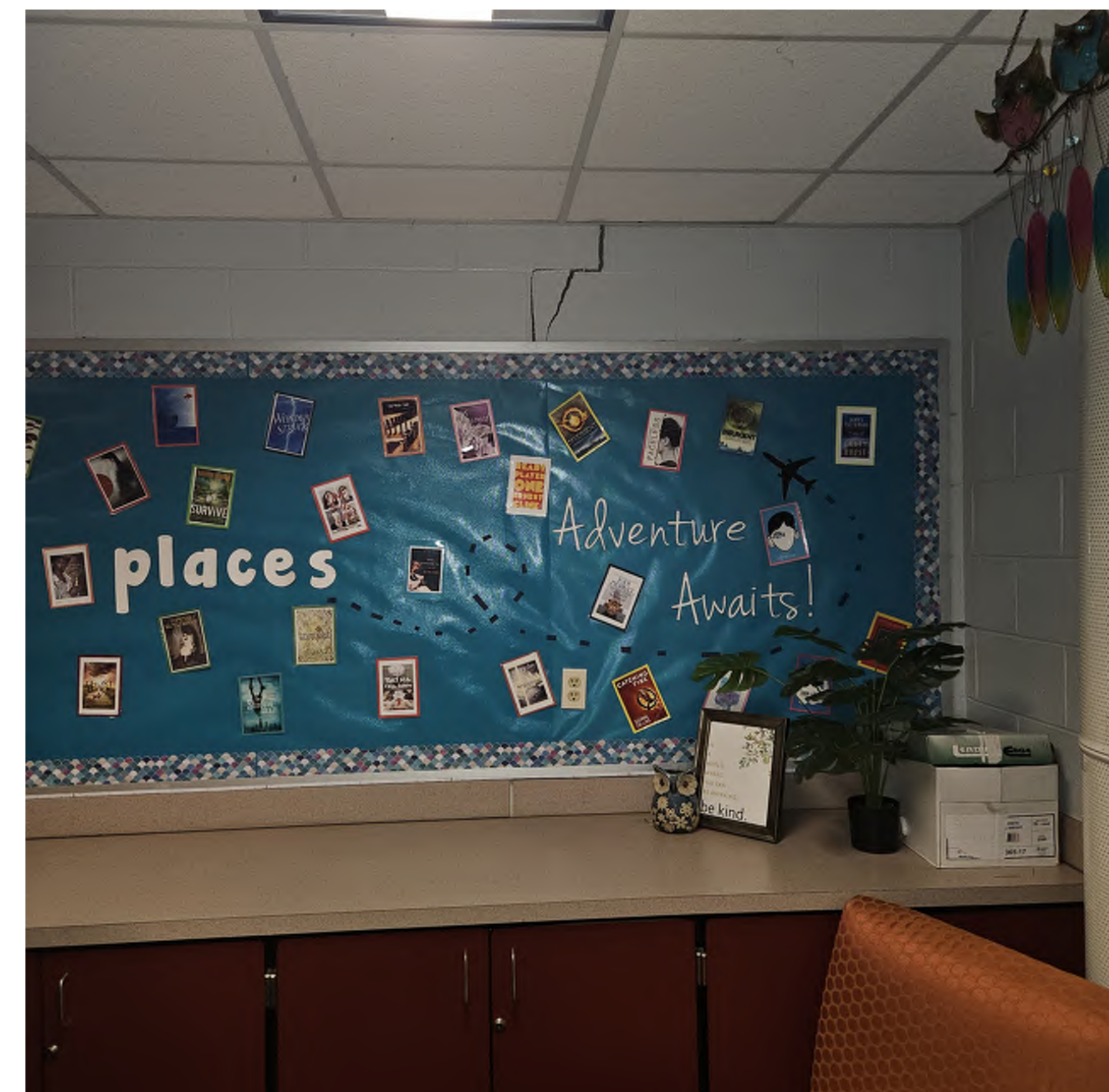
6 G100 EXISTING CRACKED CMU / TACKBOARD
