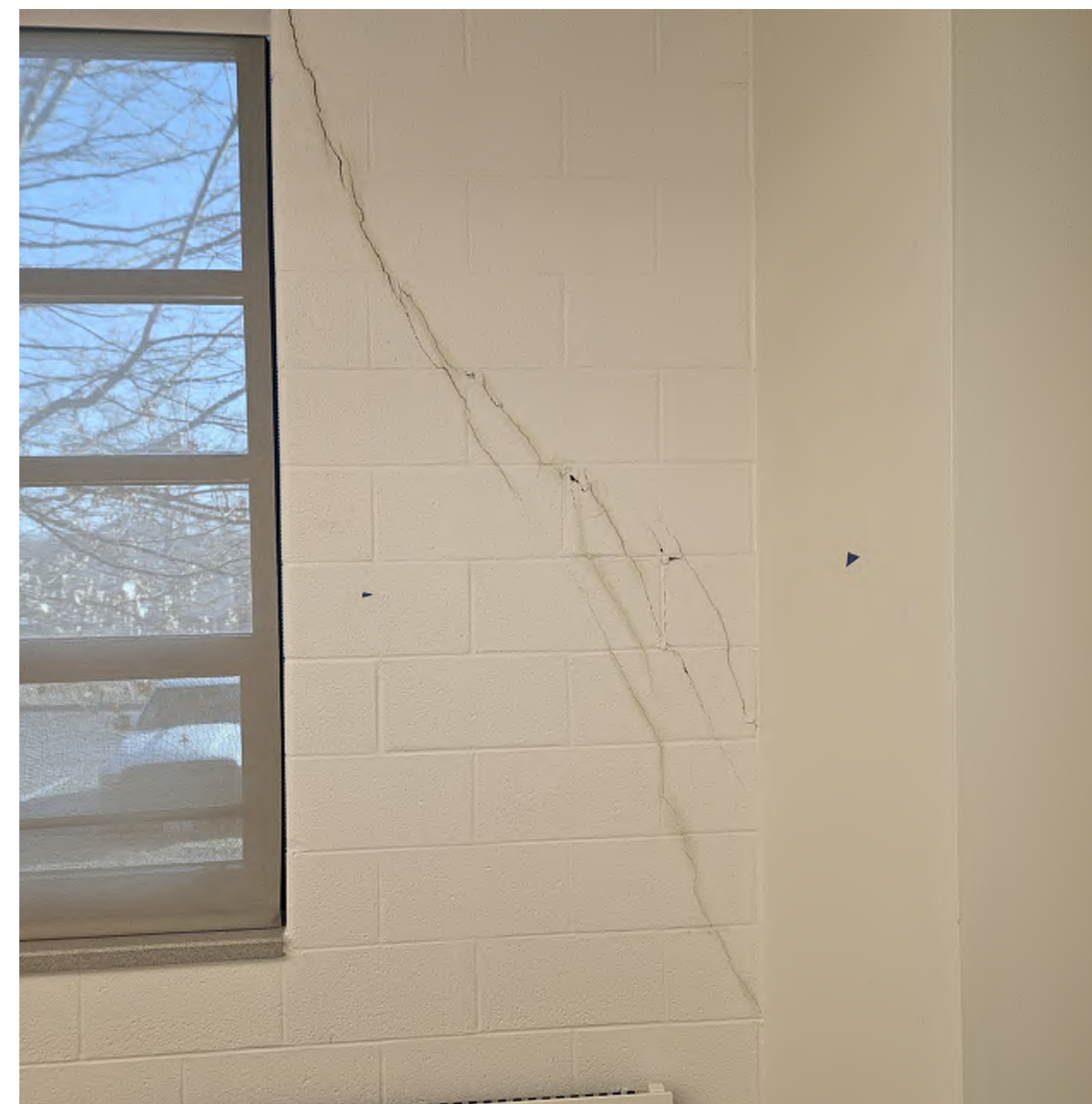
5 G125 EXISTING CRACKED CMU
