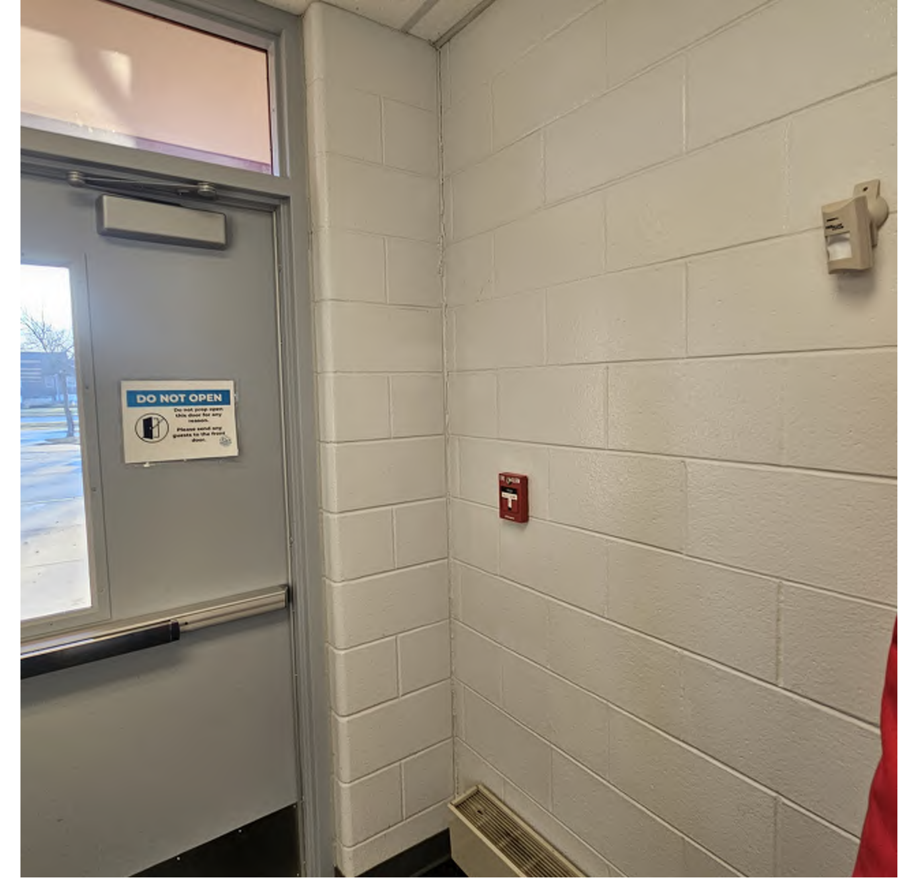
6 G110 EXISTING CRACKED JOINTS
