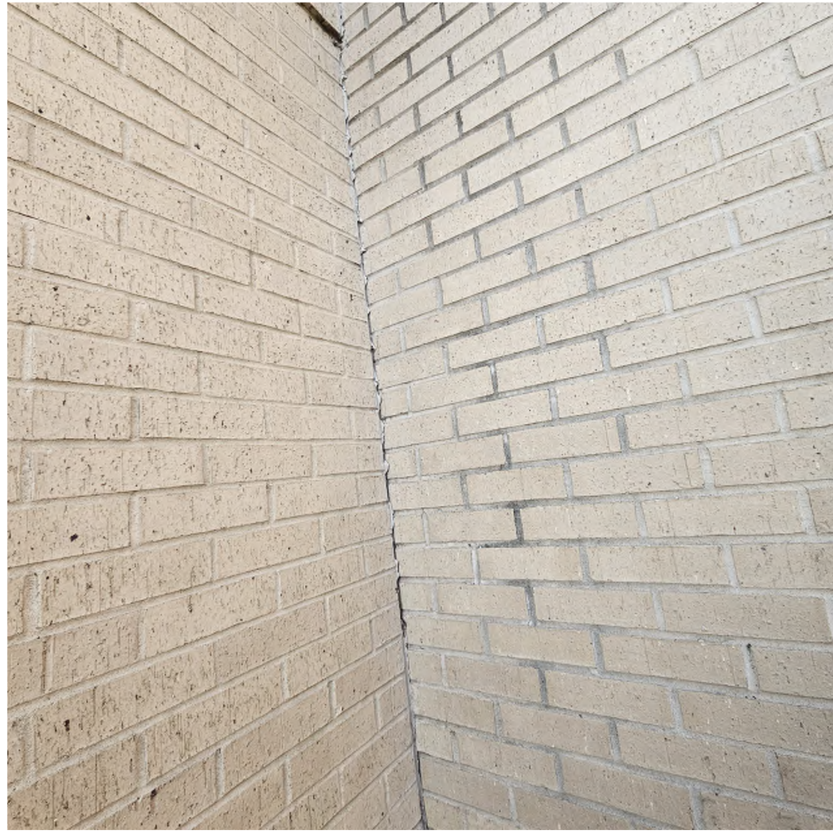
1 G110 EXISTING CORNER CRACKED JOINT
