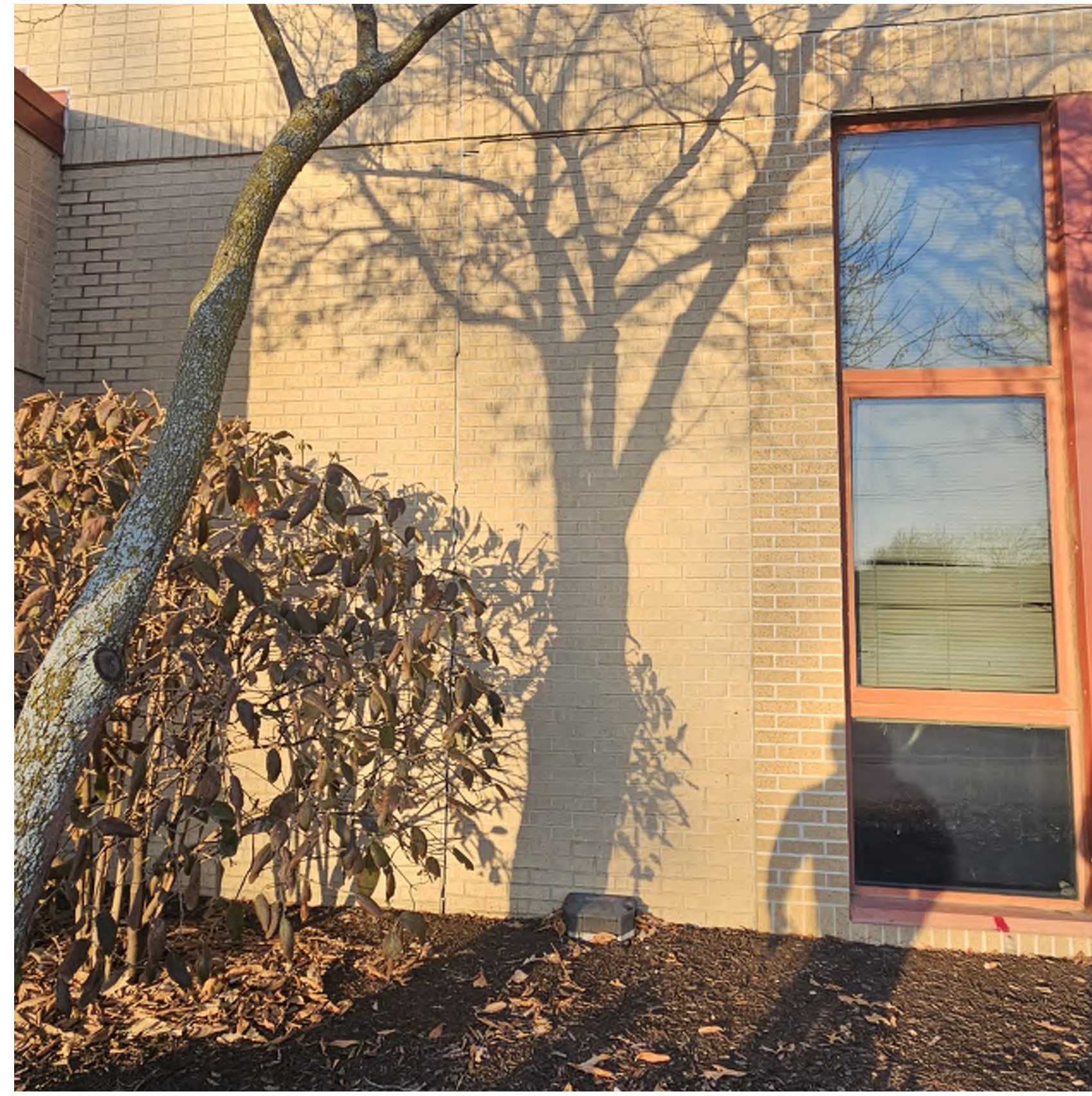
2 G110 EXISTING CRACKED BRICK/JOINTS
