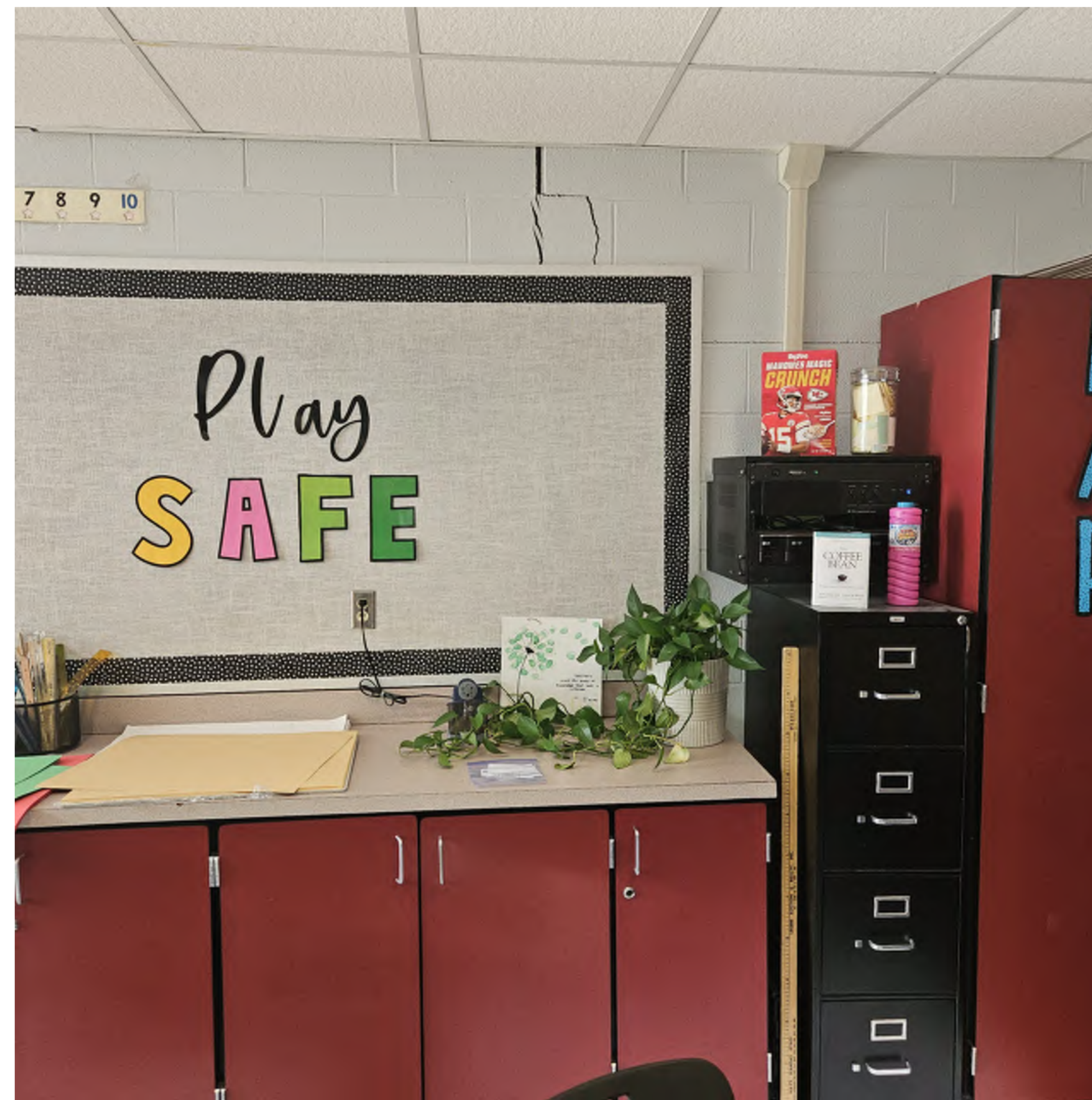
5 G100 EXISTING CRACKED CMU / TACKBOARD
