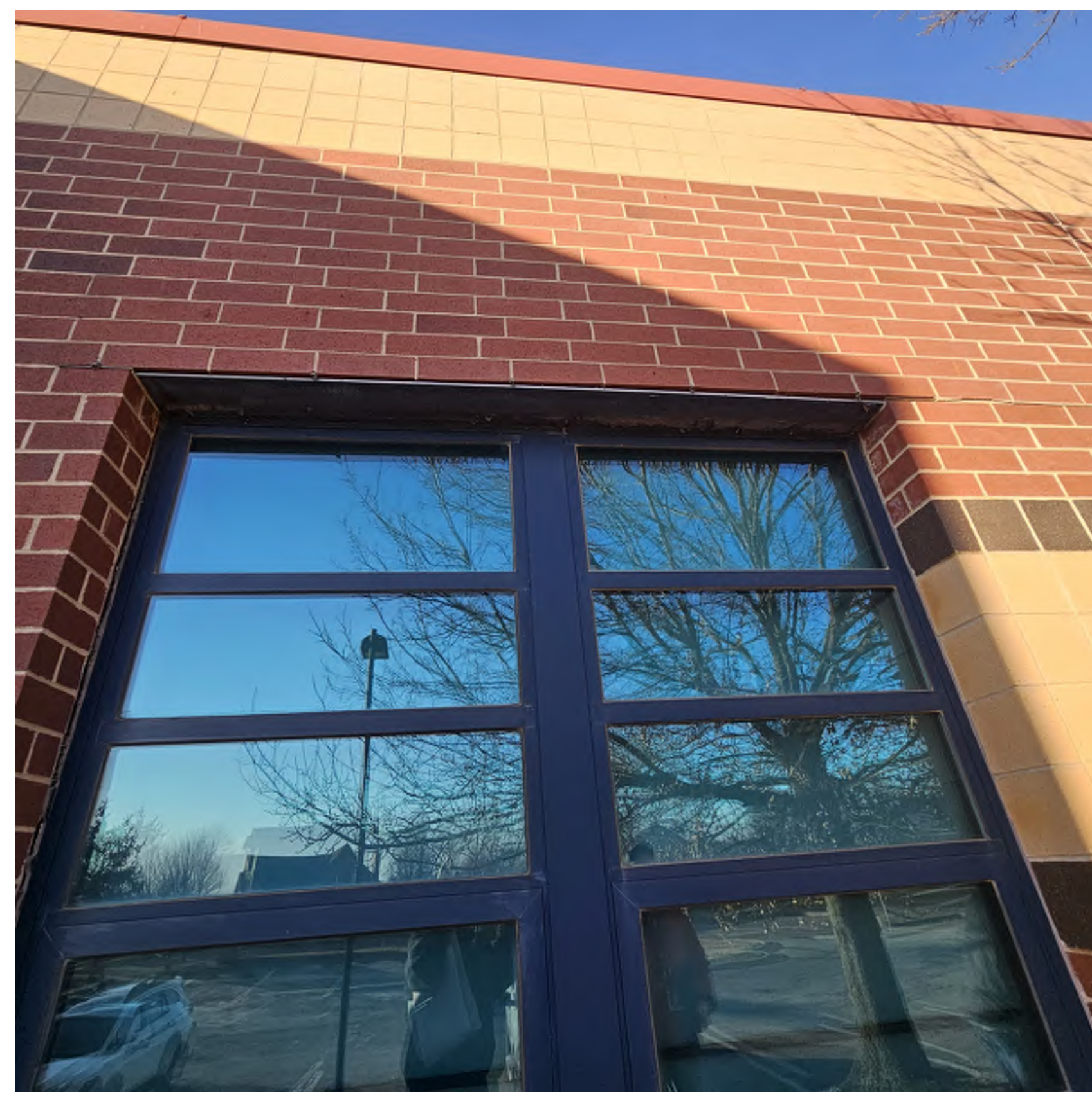
5 EXISTING TYPICAL WINDOW CONDITION G120
