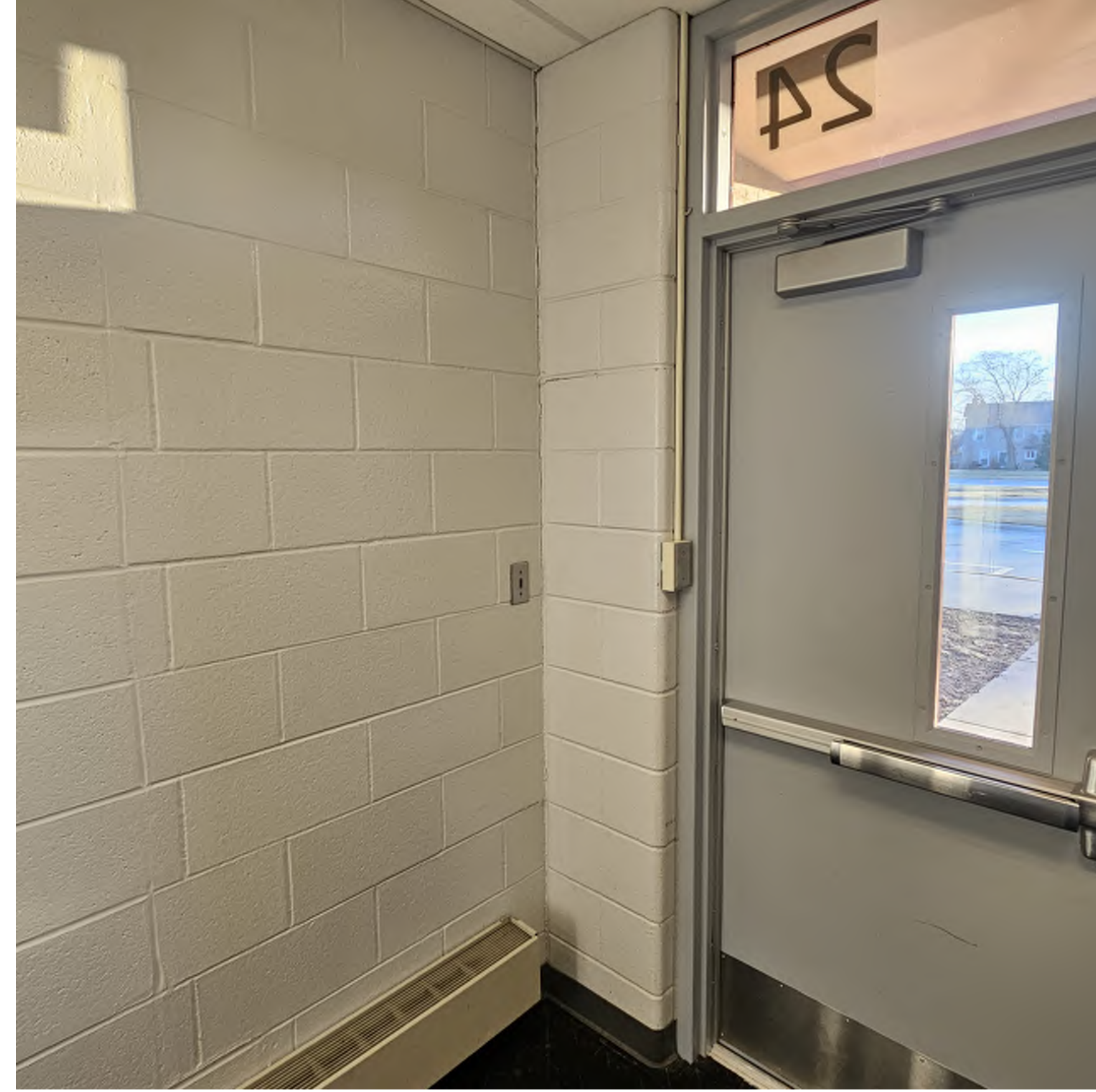
5 G110 EXISTING CRACKED JOINTS
