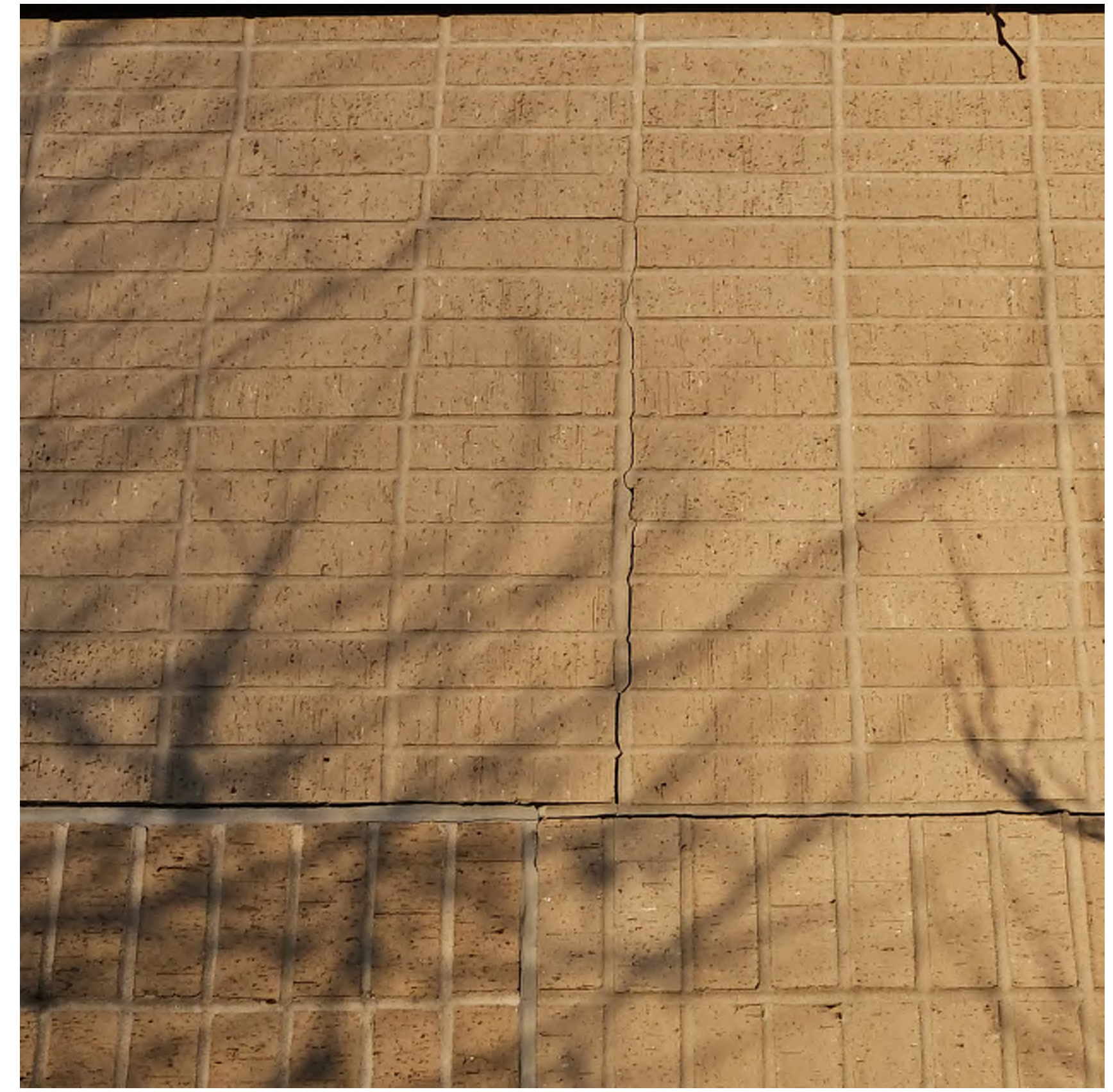
3 G110 CRACKED JOINTS ABOVE WINDOW
