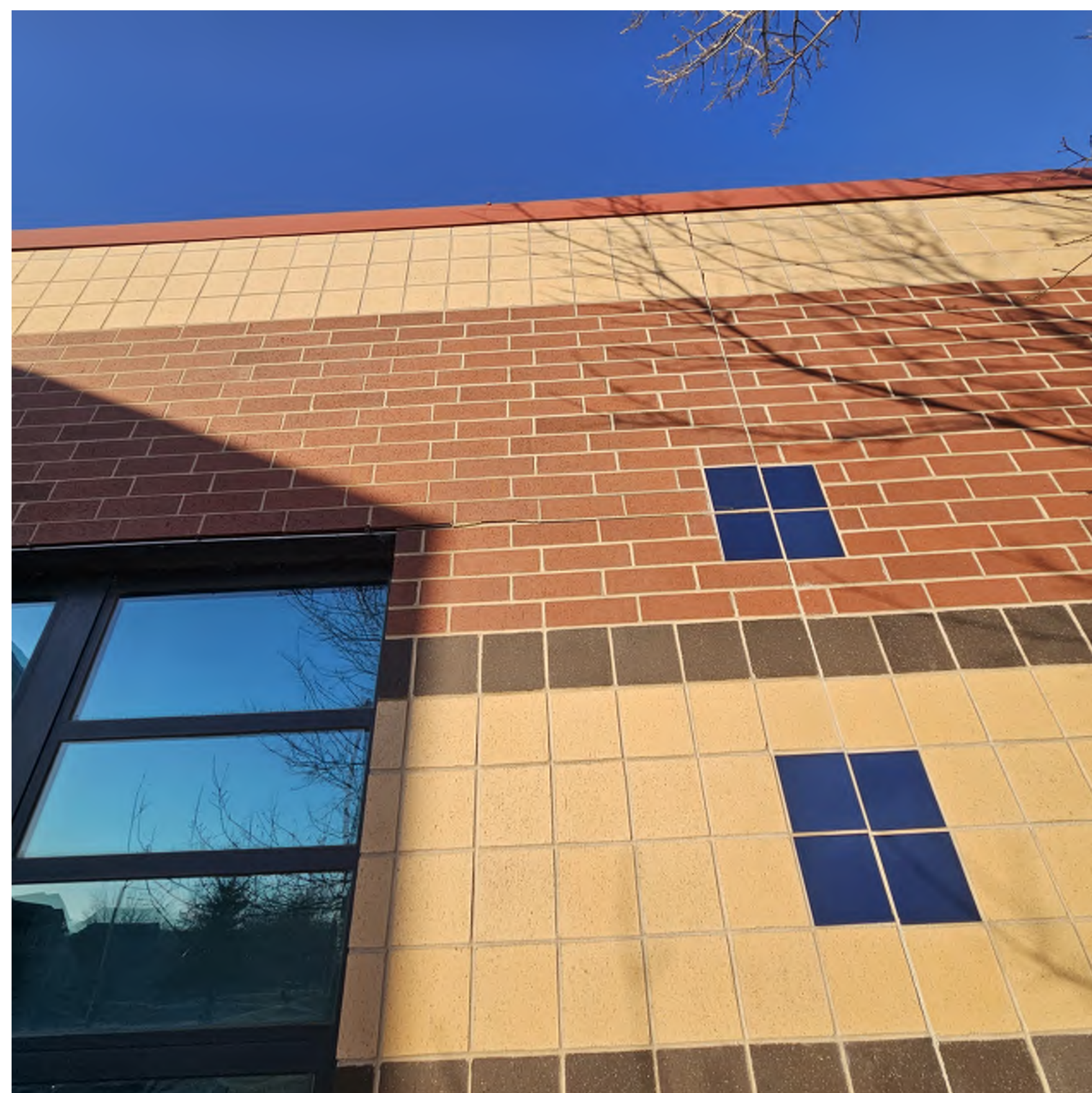
4 EXISTING CRACKED MASONRY JOINTS G120
