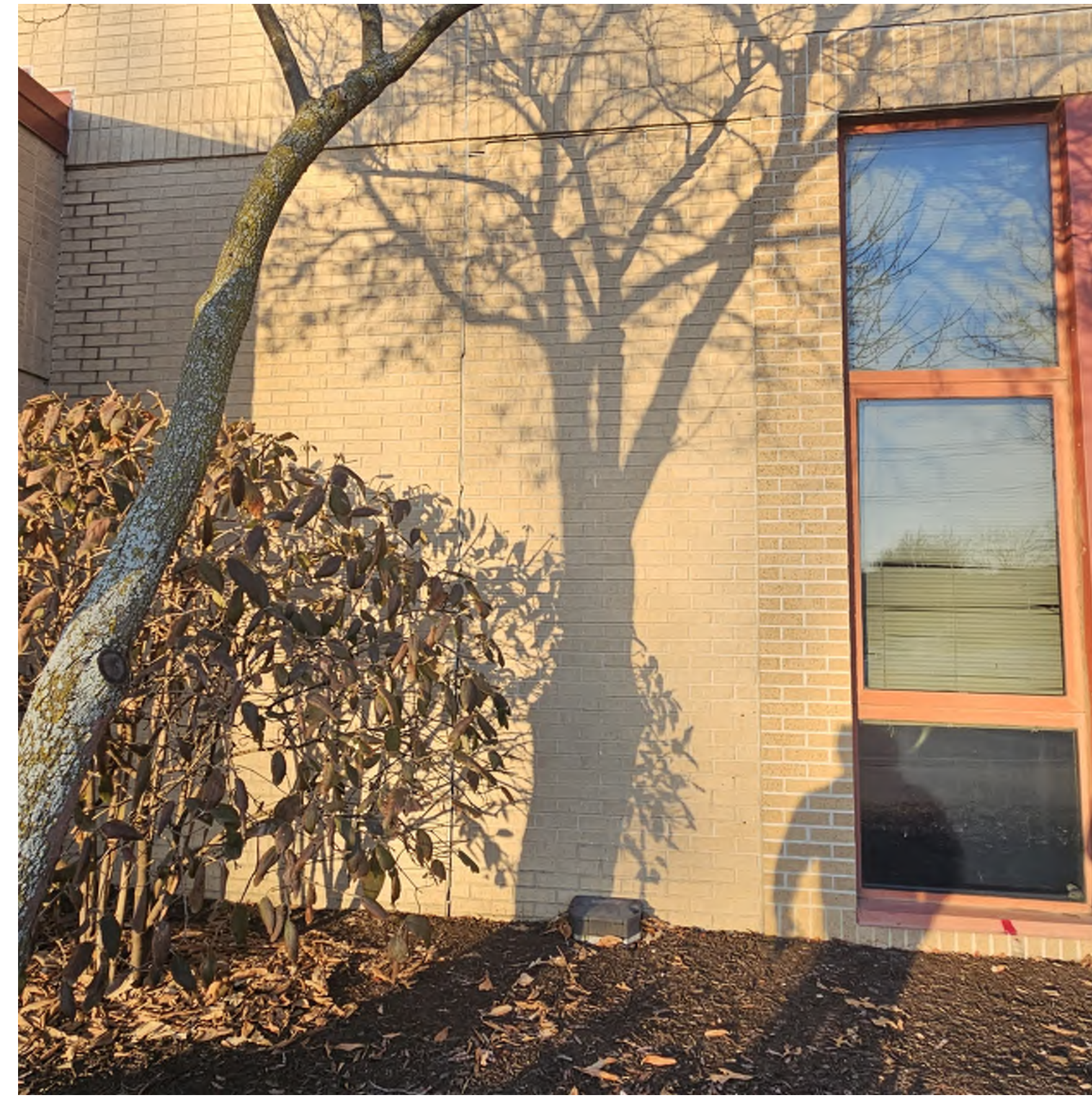
2 G110 EXISTING CRACKED BRICK/JOINTS
