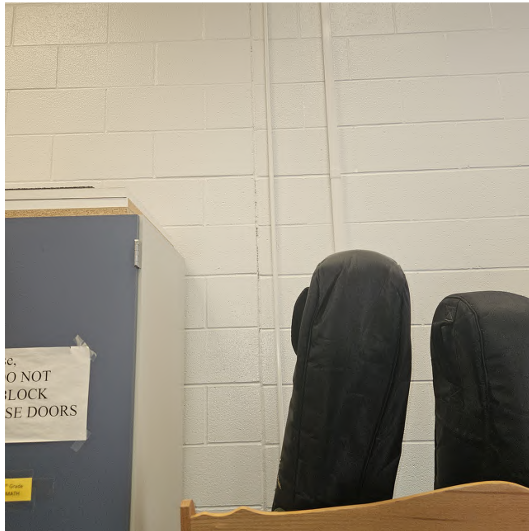
4 G111 EXISTING CRACKED CAULKING JOINT
