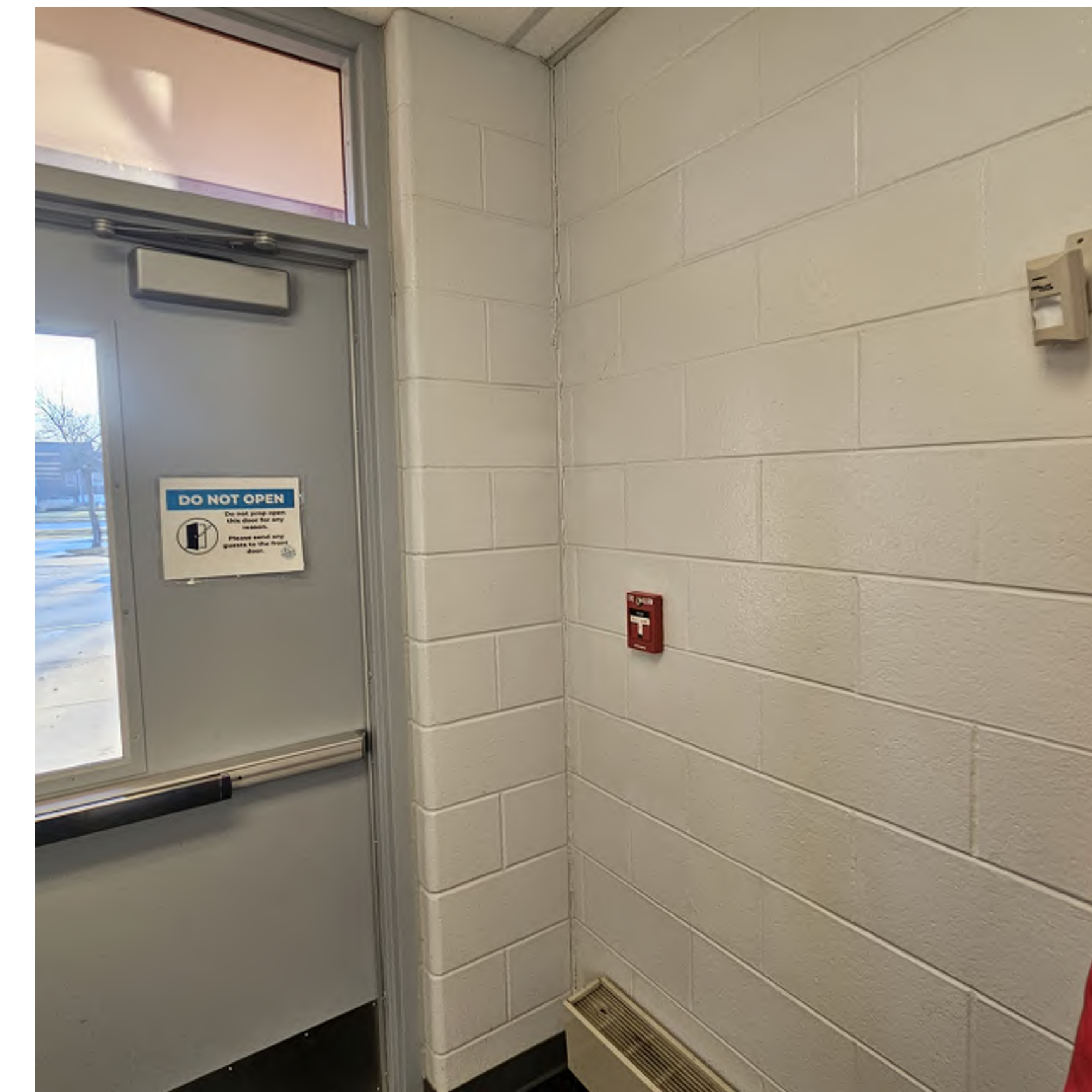
6 G110 EXISTING CRACKED JOINTS
