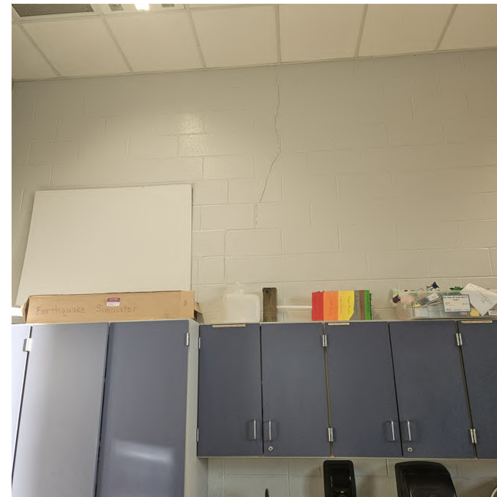
6 G111 EXISTING CRACKED CMU & JOINTS
