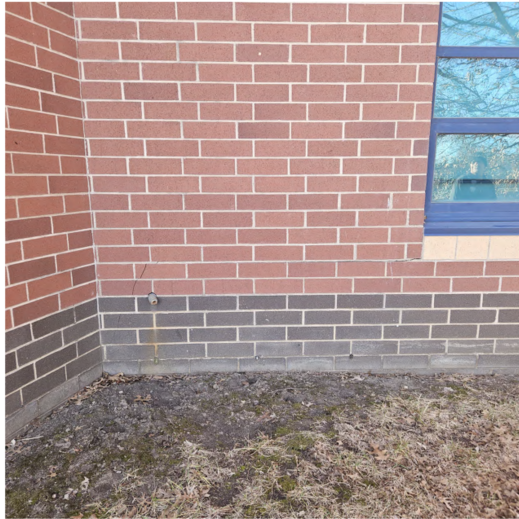
1 EXISTING CRACKED FACE BRICK/JOINTS
