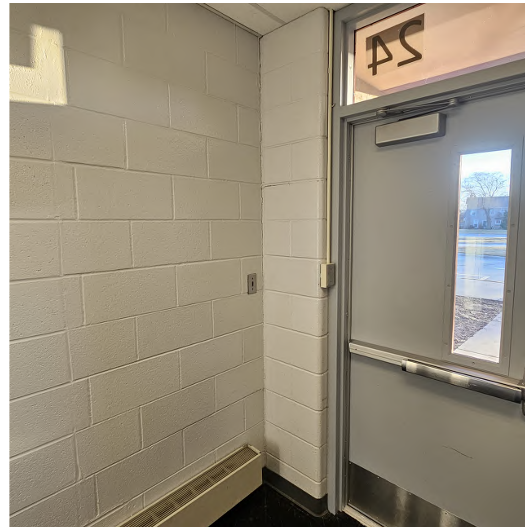
5 G110 EXISTING CRACKED JOINTS
