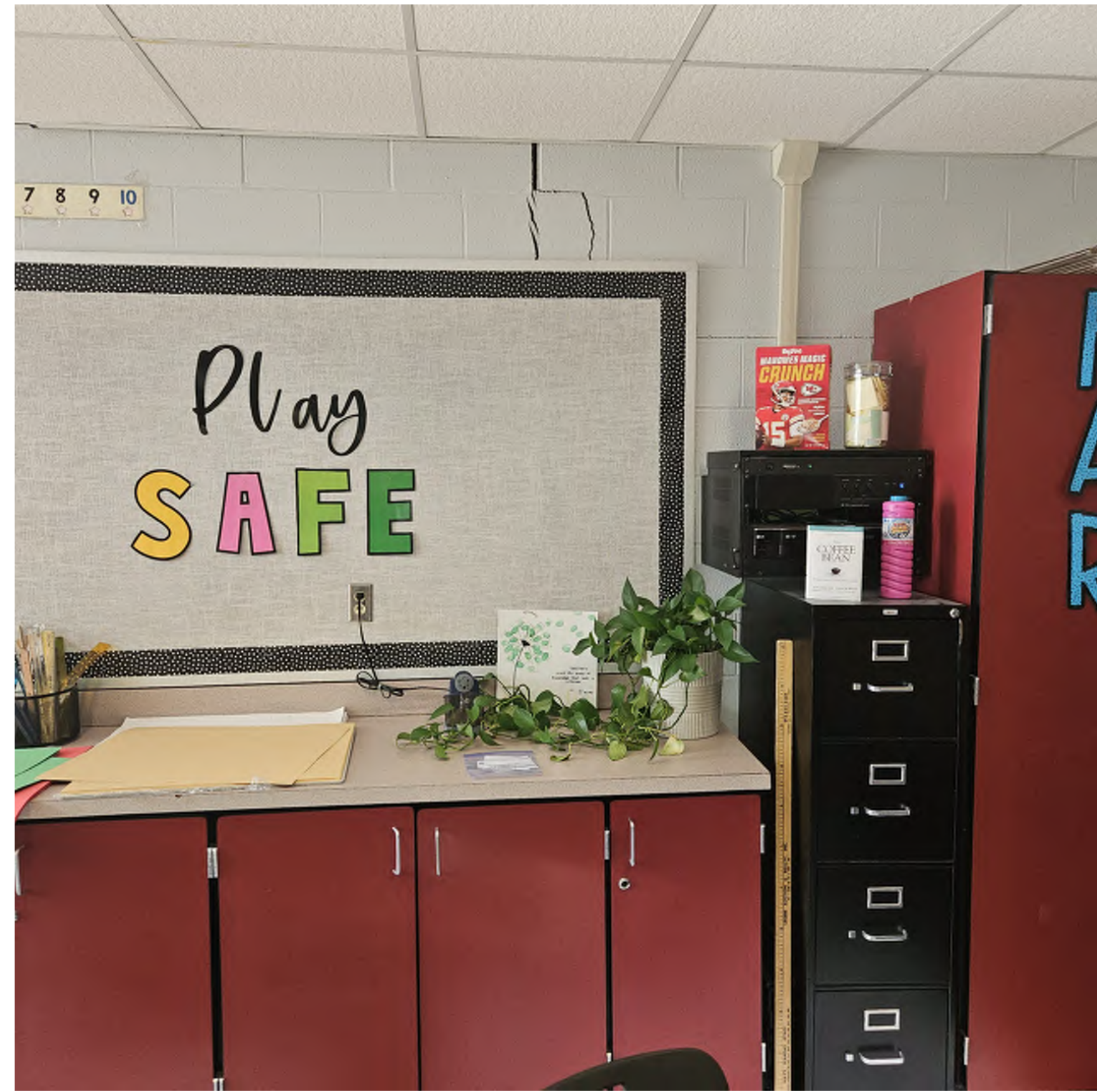
5 EXISTING CRACKED CMU / TACKBOARD G100
