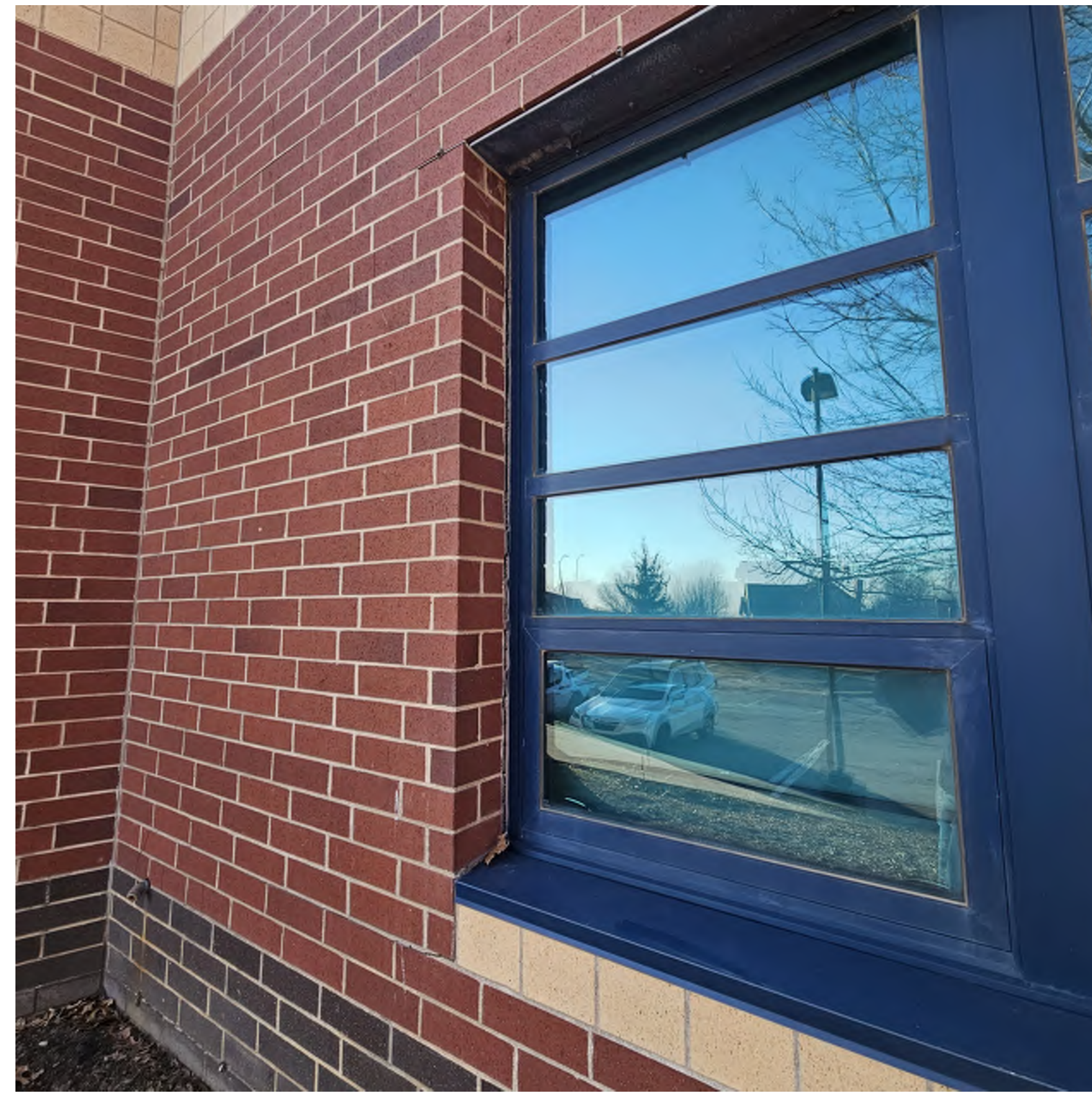
2 EXISTING TYPICAL WINDOW CONDITION
