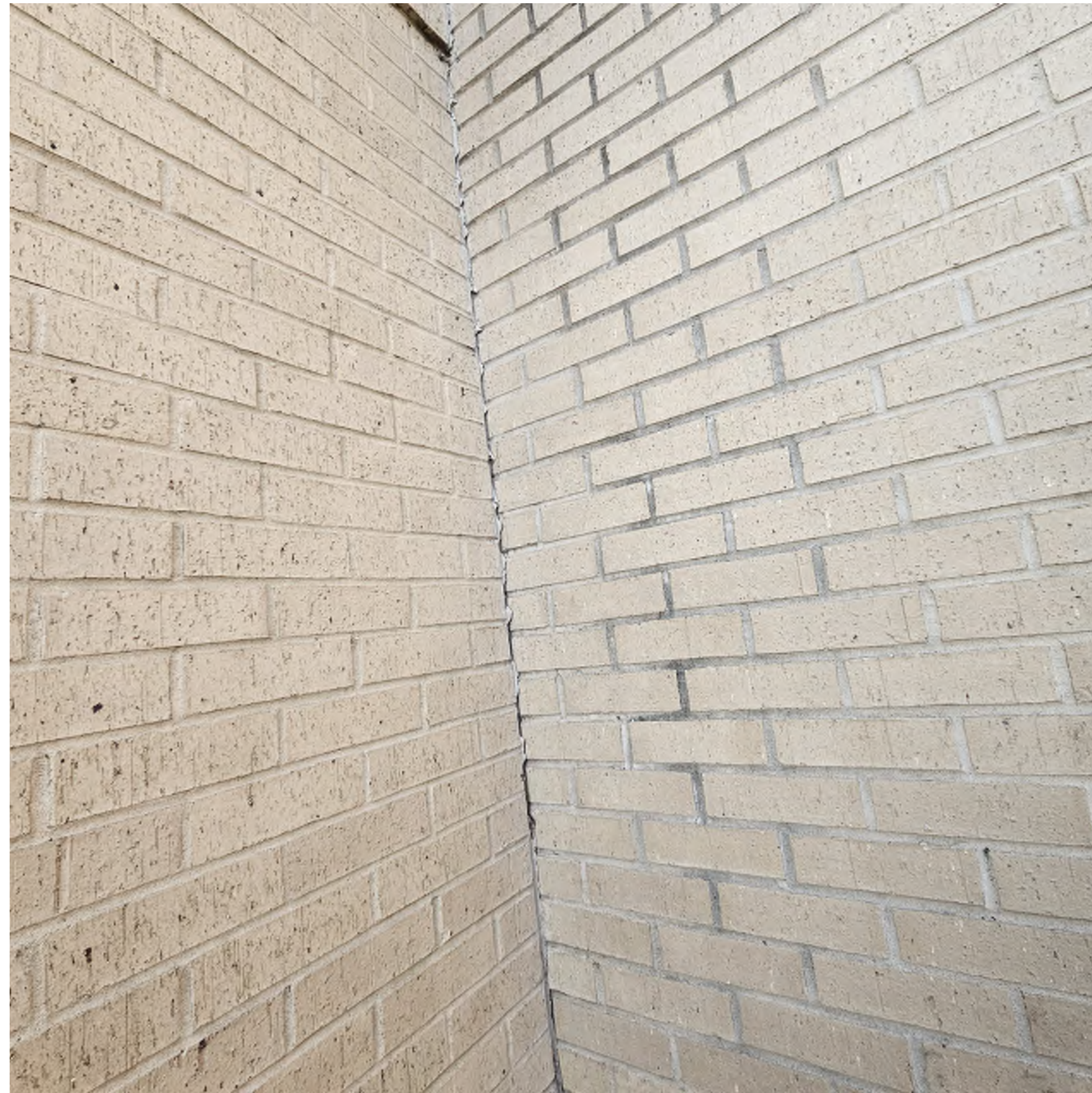
1 G110 EXISTING CORNER CRACKED JOINT
