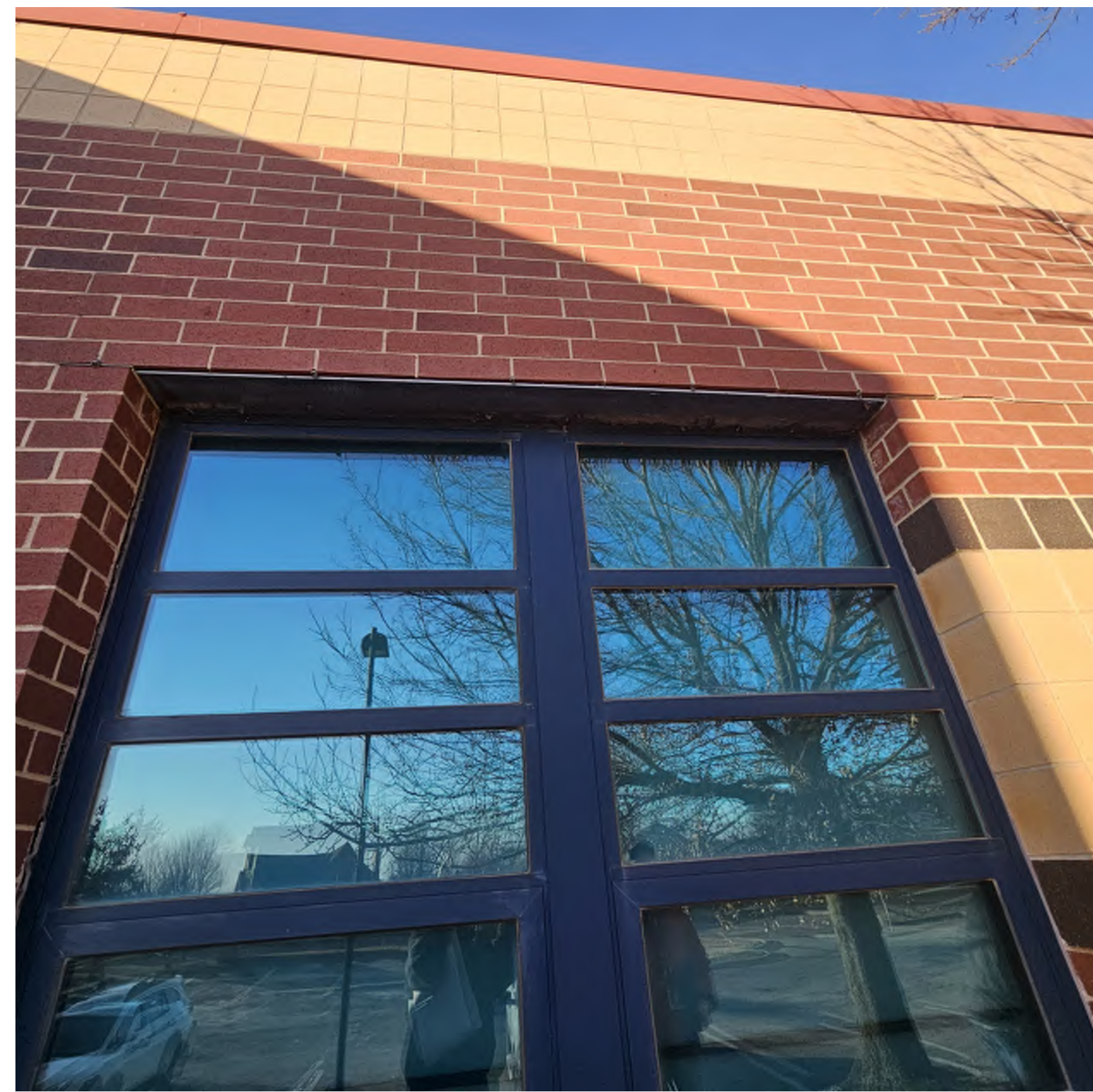
5 EXISTING TYPICAL WINDOW CONDITION
