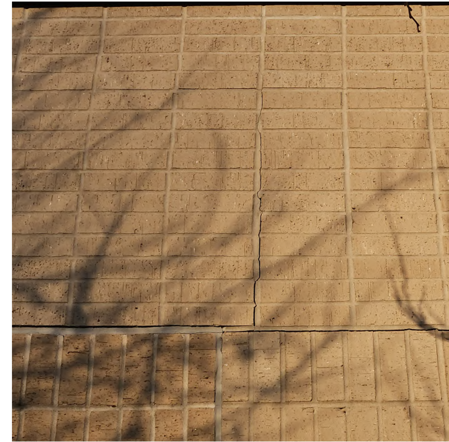
3 G110 CRACKED JOINTS ABOVE WINDOW
