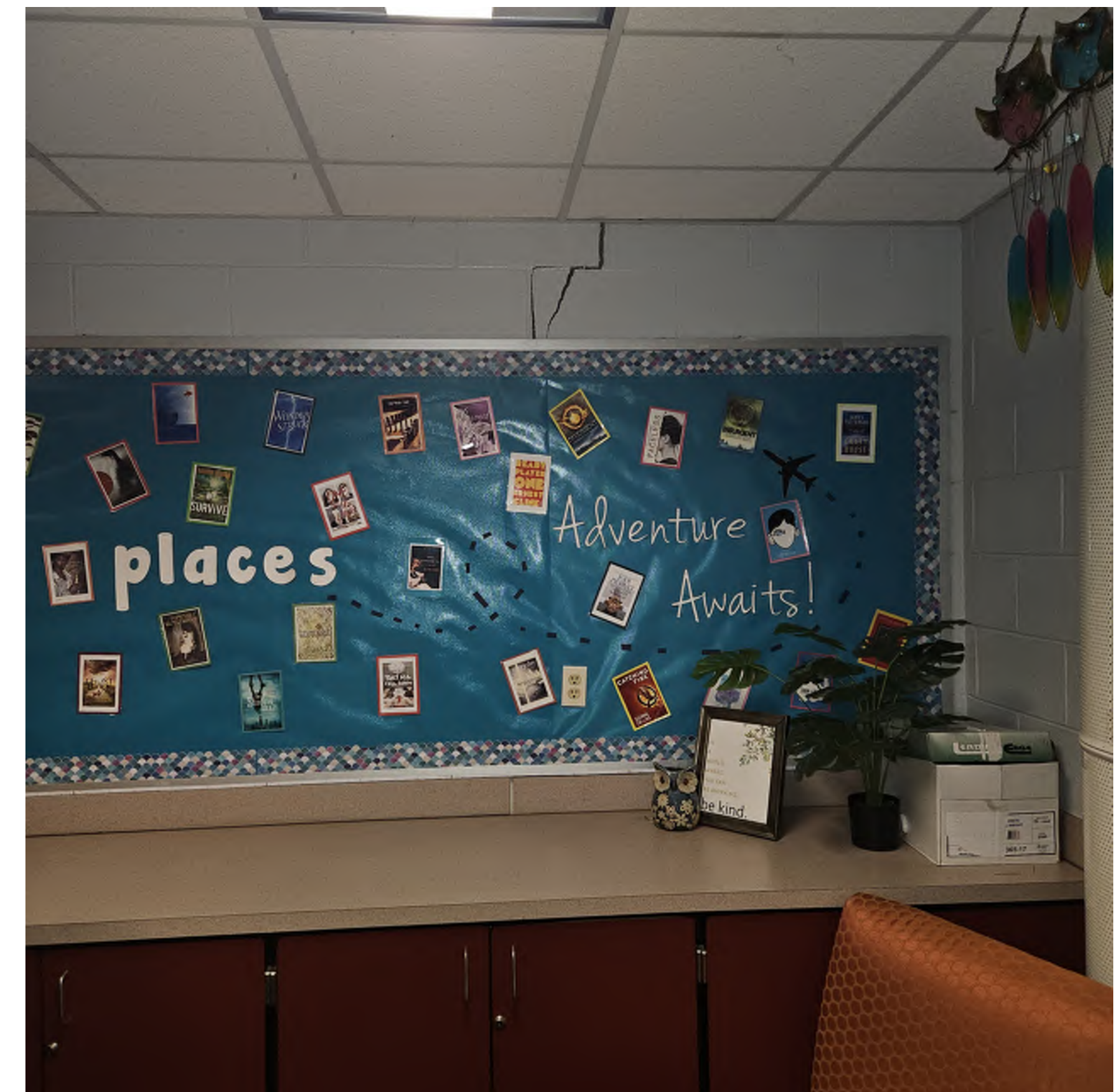
6 EXISTING CRACKED CMU / TACKBOARD G100
