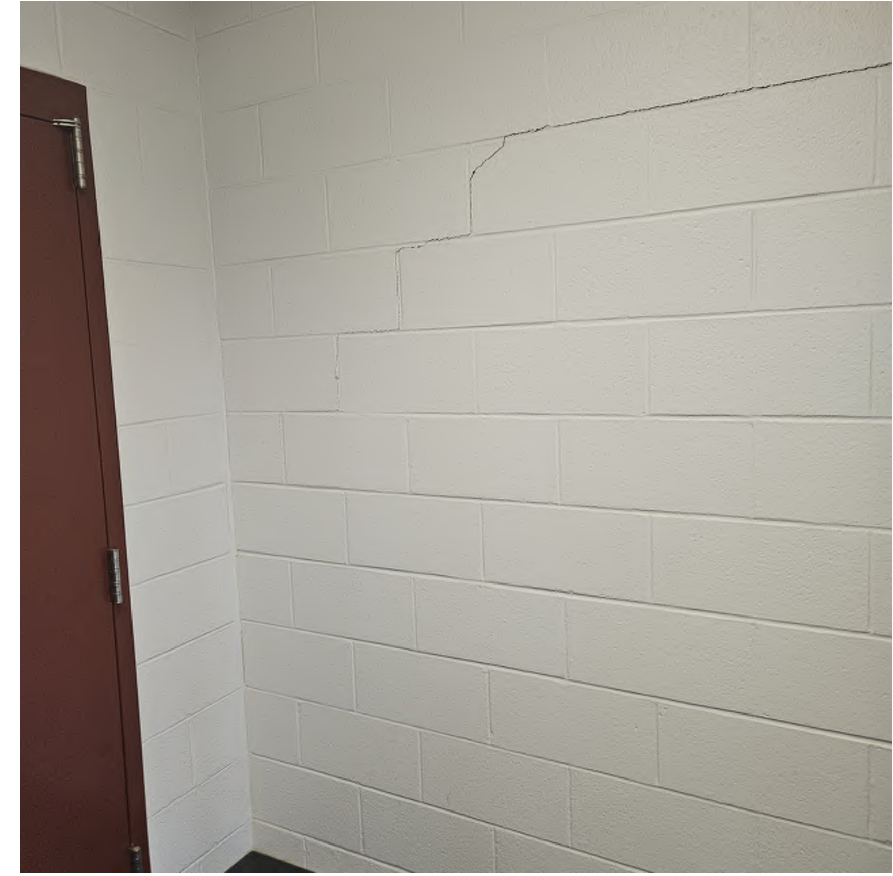
3 EXISTING CRACKED MASONRY G100
